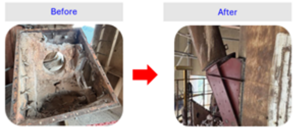
New design of splash box implemented at kiln #3, SCCTH
