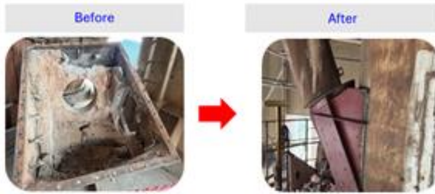
New design of splash box implemented at kiln #3, SCCTH
